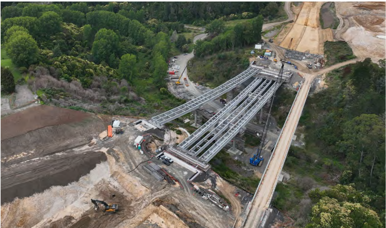
Te Rangi tua nehe / Minden Gully area of the Takitimu North Link Stage 1 site, at Te Puna. Takitimu North Link will provide an efficient, reliable and safer route between Tauranga and Ōmōkoroa.
